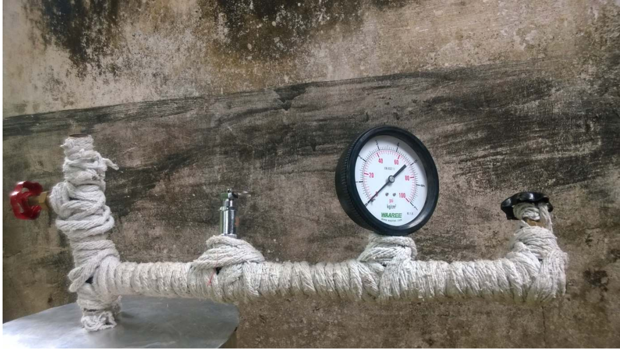
Fig: Steam flow regulation unit
